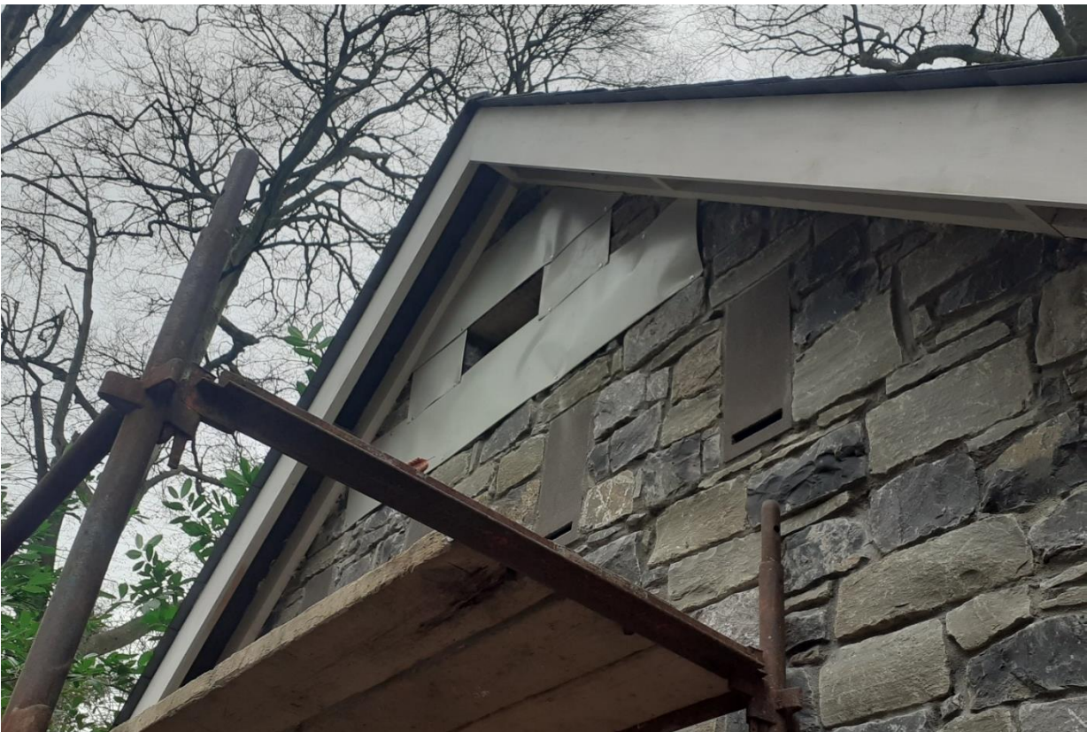
Plate 5: Example of predator proofing on external wall around entrance point of bat house.
